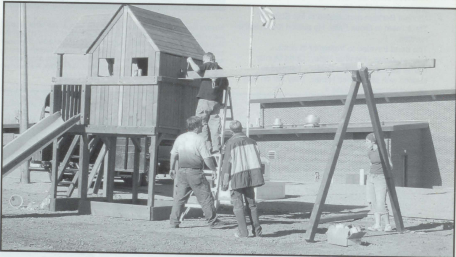
Mr. Brian Jorgensen, industrial arts teacher, works with students Lance Ring, Matt Karges, and Lindsay Zeigler as they construct the new playground equipment for the elementary kids. The money for the equipment came from several sources. A grant from the Greater Missouri Community Development provided $2,350 for the project. Holly Cahoy and Tari London headed an effort to raise money with a raffle. The PTSO also raised money with a tailgate party. Mrs. Marsha Risseuw of Modern Woodmen of America matched $500. The Colome School Board provided the rest of the money.
